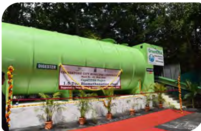
Biomethanation Plant at Coimbatore City Municipal Corporation in Ward 69 under CapaCITIES Project by ICLEI South Asia, 2019
